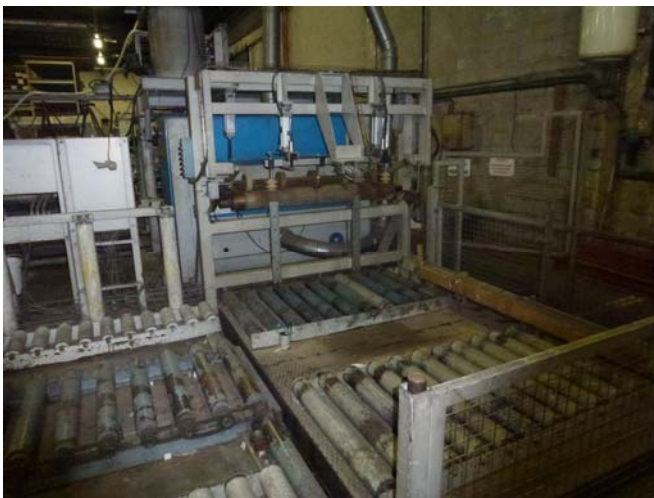
Raw board stack in-feed
