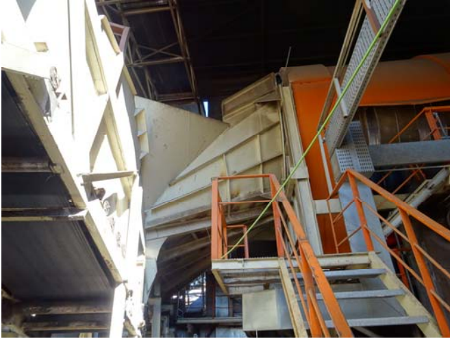
Log belt conveyer
