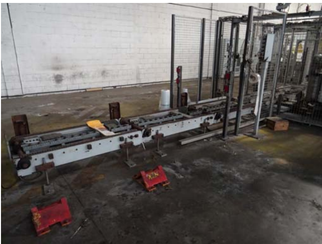
Infeed chain conveyors
